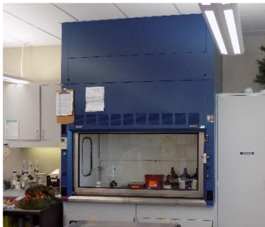
Chemical Fume Hoods
