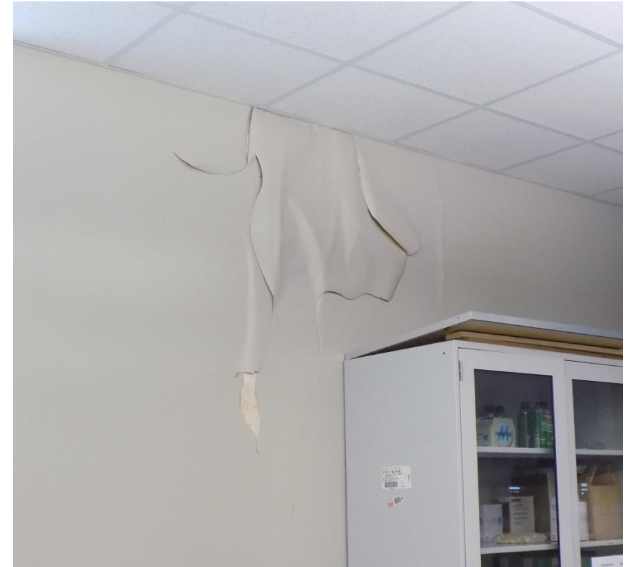
Water Damage to Walls from Roof Leaks
